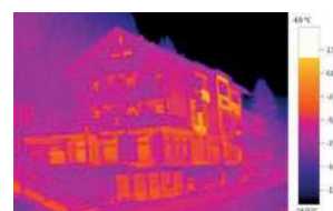
Thermal image with ScaleAssist
